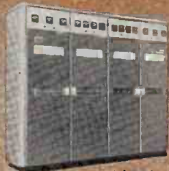
2 kw, for VHF Type TT-2AL/H (All Air-Cooled)
