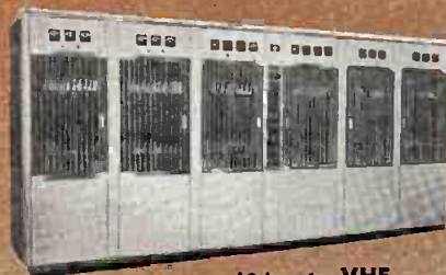
10 kw, for VHF Type TT-10AL/H (All Air-Cooled)
